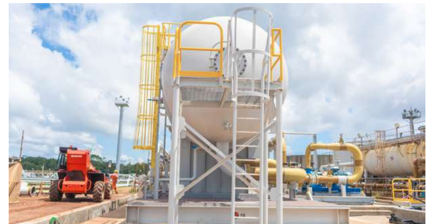
ISF-3 unit at Gamba Terminal in November 2023.]
